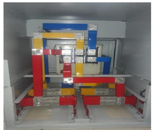
LT BUSBAR FITTINGS
